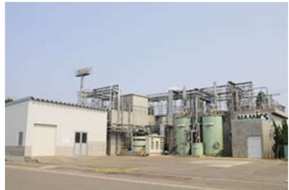
Wastewater treatment facilities (Head Office/Factory)
