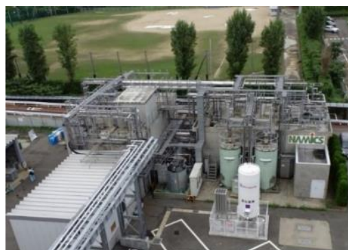
Wastewater treatment facilities (Head Office/Factory)
